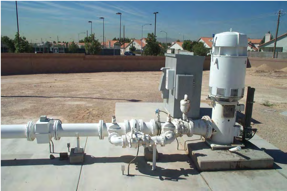
Figure 2 Converted Dual Use ASR Well (LVVWD, Well 33)
