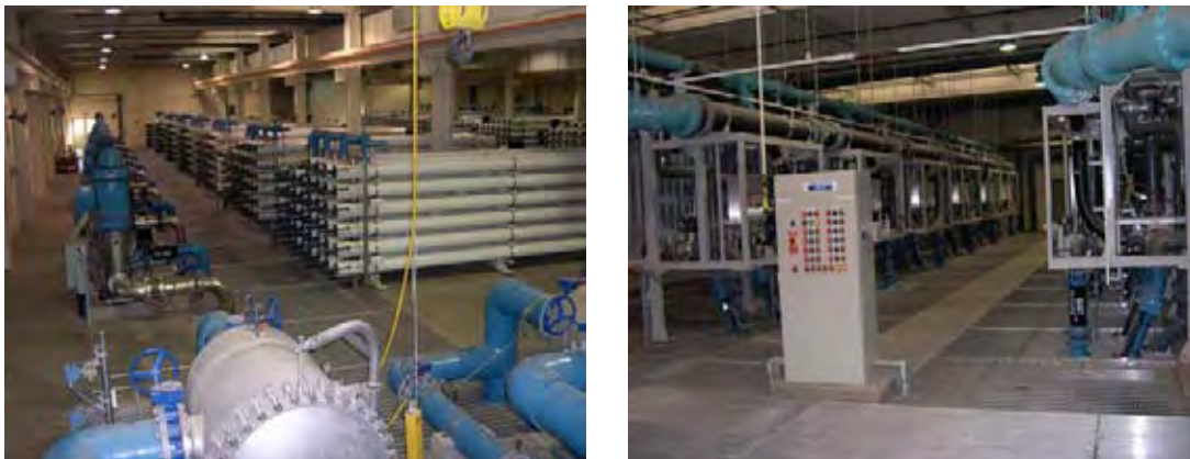
Figure 2: Microfiltration and Reverse Osmosis Trains (Pugh, 2006)
