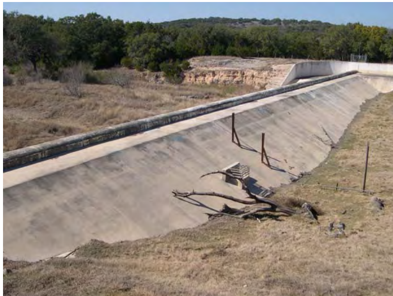
AA Verde Creek Recharge Dam (February 2006)
