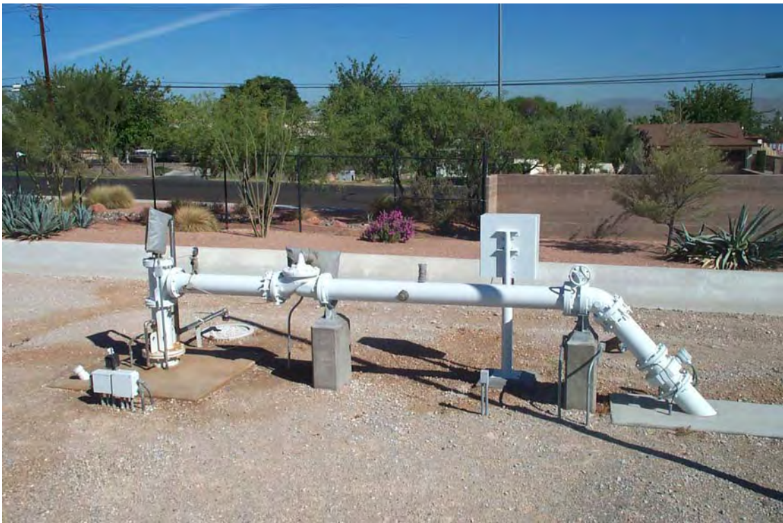
Figure 3 Dedicated Recharge Only Well (LVVWD, Well AR-1)
