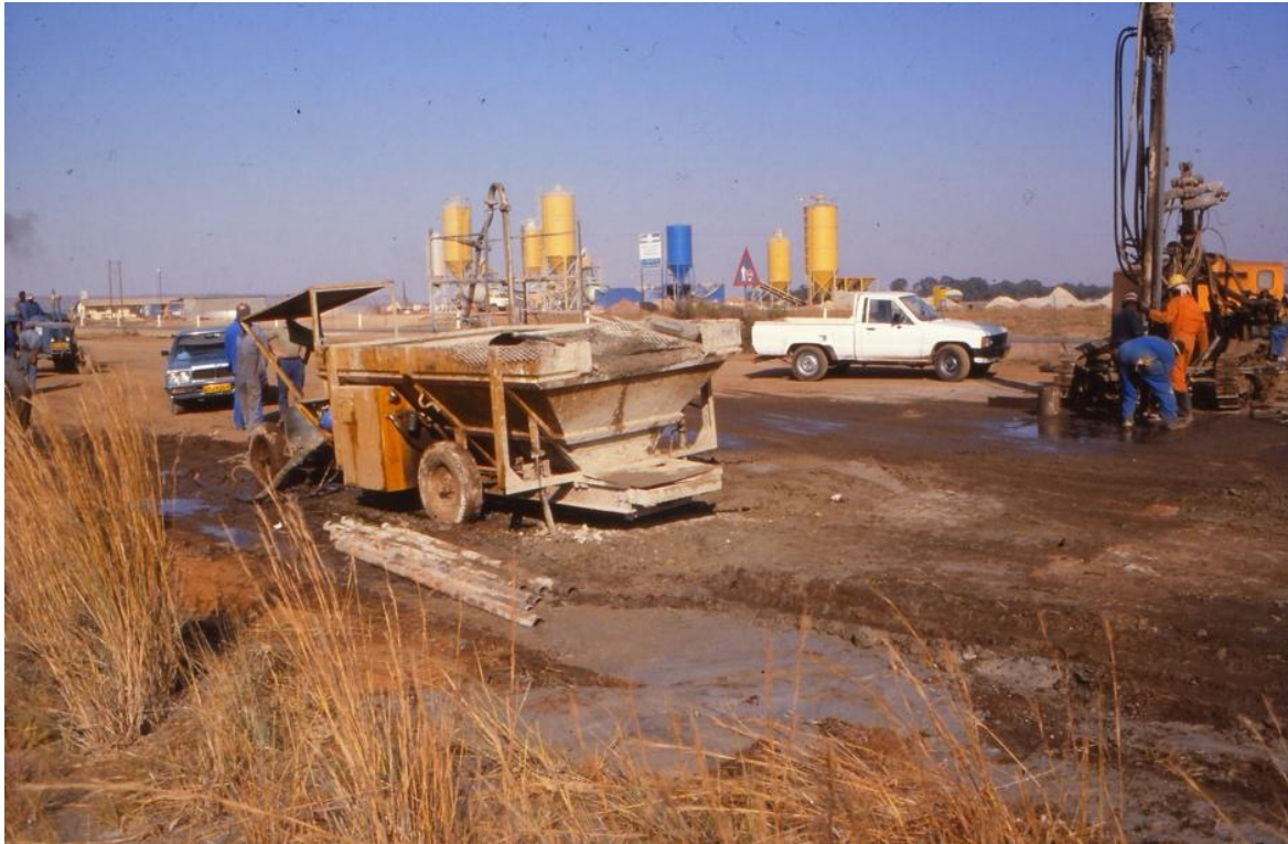
Figure 67 - Grouting operation along the closed left lane of the dual carriageway (Photograph by van Rooy).
