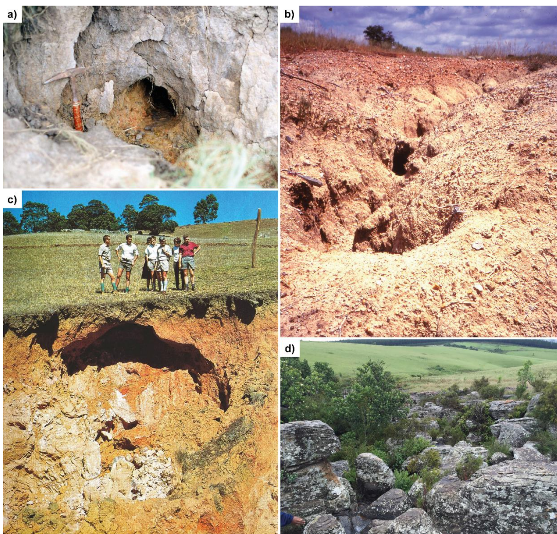
Figure 14 - Examples of karst features in non-soluble rocks: a) pseudokarst suffusion in Namaqua-Natal Province Granitoids of Bizana South Africa (photograph by Dippenaar, 2002), b) pseudokarst piping daylight in Nebo Granite of Lebowakgomo, South Africa (photograph by van Rooy, 1992), c) pseudokarst sinkhole Mpuluzi Granitoid Batholith of Hlatikulu, Eswatini (photograph by Brink, 1979) and d) pseudokarst in Black Reef Quartzite of Kaapschehoop, South Africa (photograph by Dippenaar, 2016).
