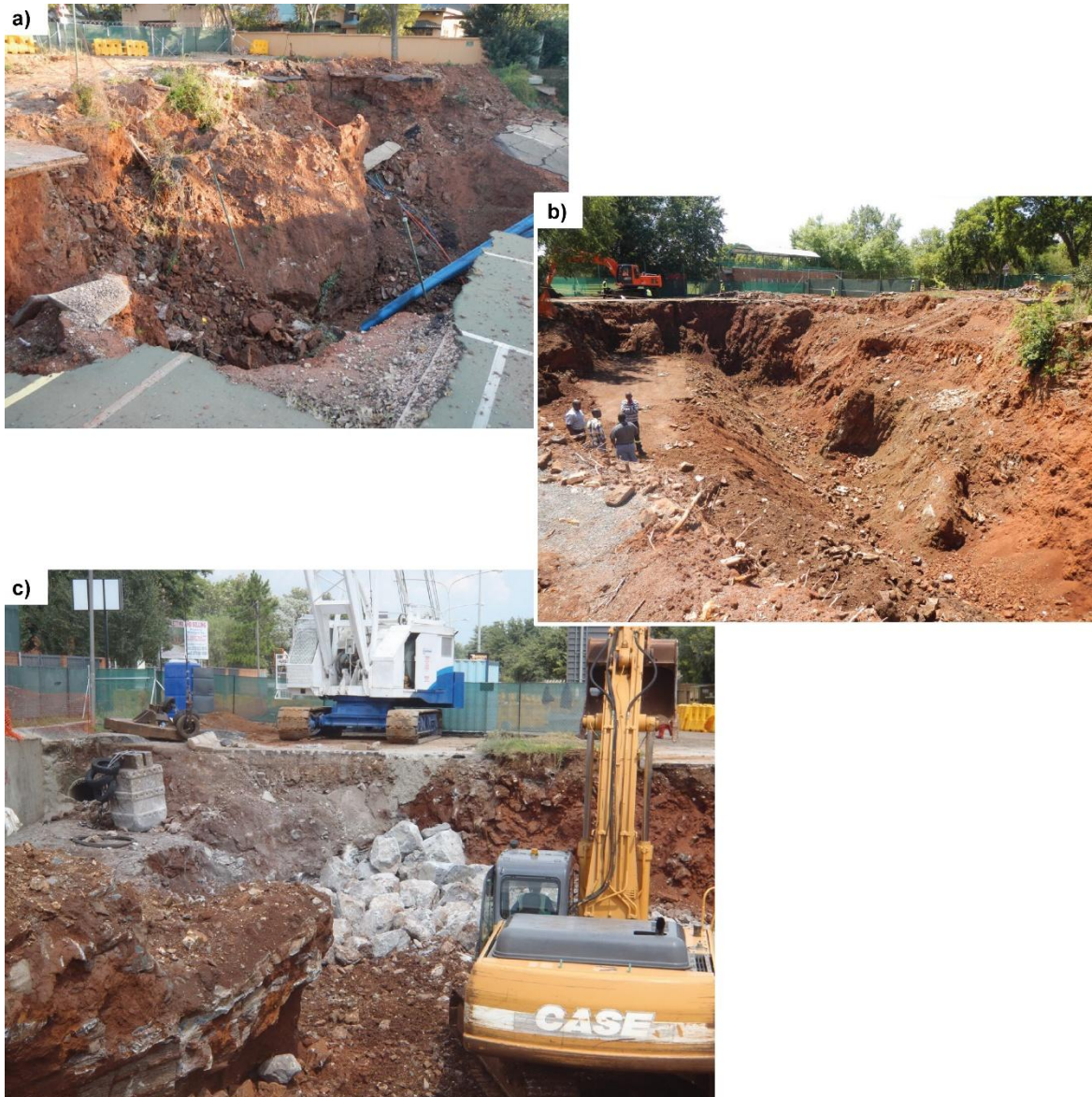
Figure 60 - Illustration of the rehabilitation process: a) original sinkhole, b) excavation of slumped overburden material and c) dynamically compacted rockfill base prior to complete backfill (photographs by van Rooy).
