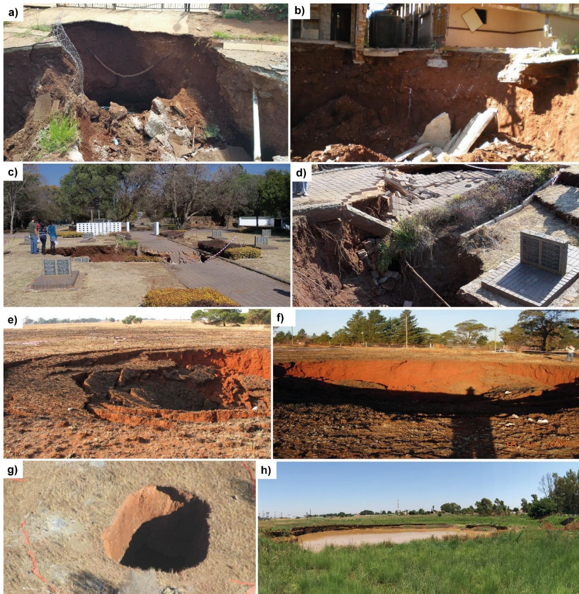
Figure 35 - Photographs of water ingress sinkholes. a) An initial 10 m diameter sinkhole increasing to b) 30 m diameter due to raveling and further erosion affecting two houses (Centurion, Pretoria, South Africa). c) and d) A sinkhole in a cemetery resulting in damage to graves (Pretoria, South Africa, 2010). e) and f) A sinkhole due to groundwater dewatering 20 m diameter in 2007 and tension cracks indicating development towards maximum size in 2017 (Bapsfontein, Gauteng, South Africa). g) A sinkhole due to deep mine dewatering in Far West Rand, South Africa (2019). h) A flooded sinkhole in Bapsfontein, Gauteng, South Africa (2019) (photographs by Dippenaar).
