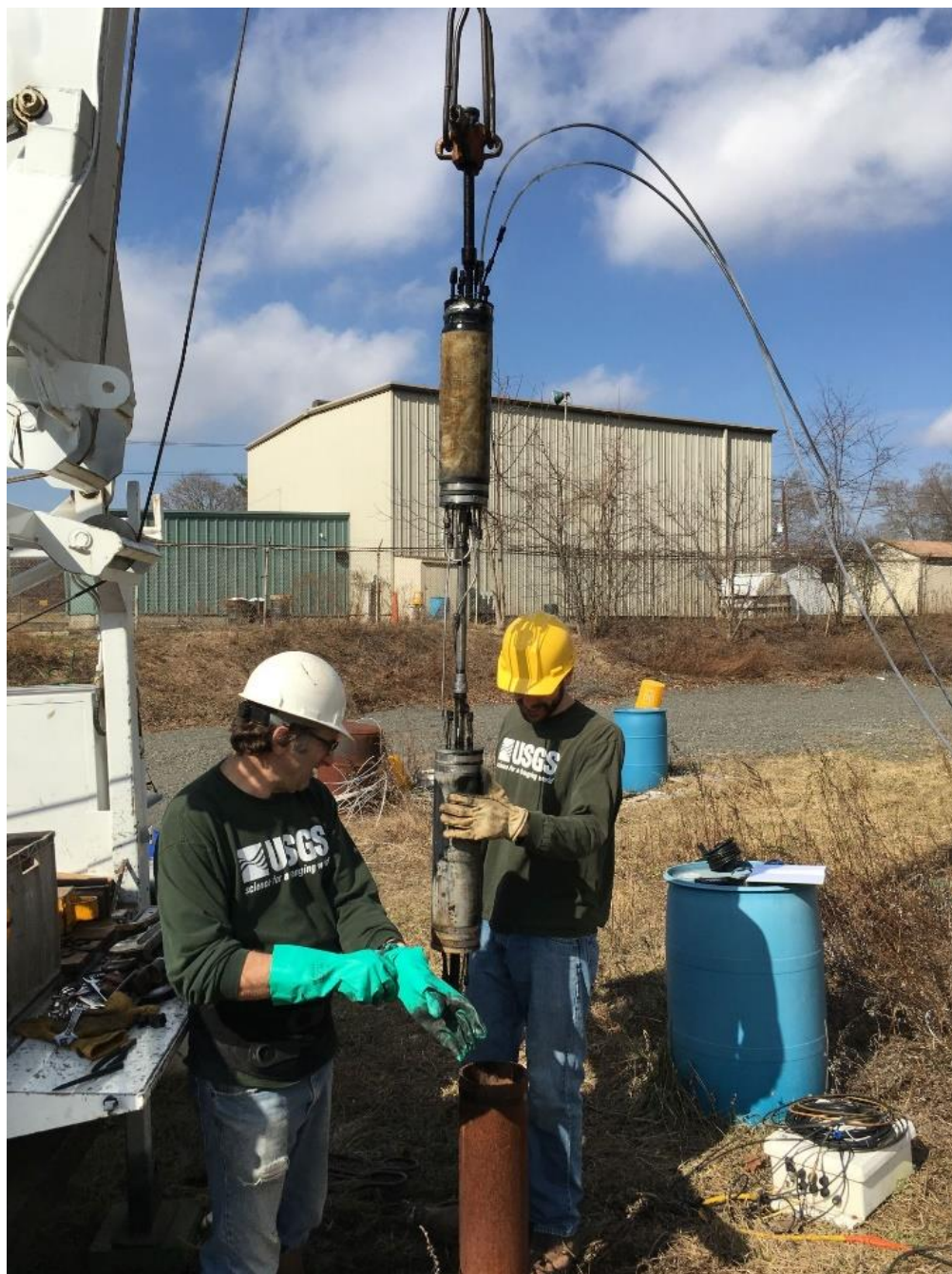
This photograph shows the installation of two packers used to isolate a section of open borehole ( http://www.usgs.gov/media/images/photograph-usgs-hydrologists-and-packers-well-testing ).
