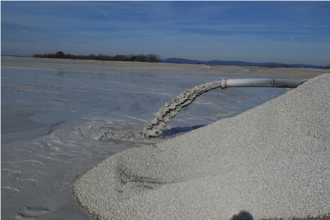
Figure 10 - Example of spigot discharge of tailings slurry from the embankment of a tailings storage facility.
