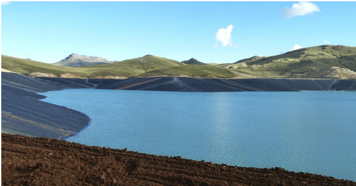
Figure 18 - Geomembrane liner installed in a tailings storage facility. At the time of this photograph, water was being accumulated in the facility for startup of mill operations.
