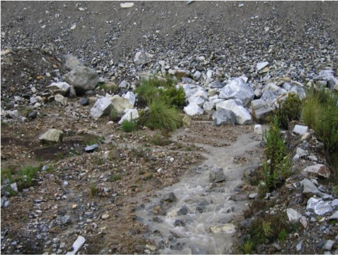
Figure 12 - Toe seepage emerging at the base of a waste rock pile.
